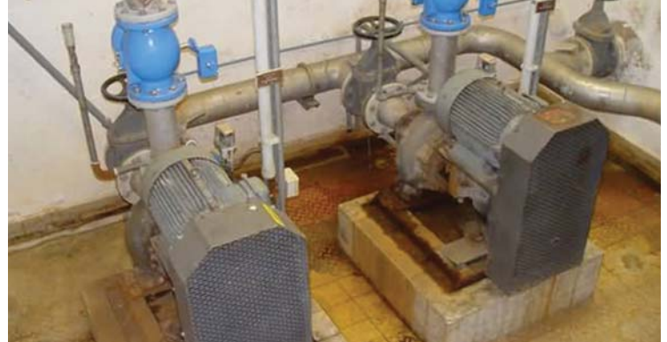
Allweiler’s optimization recommendations made it possible to eliminate these two centrifugal pumps, saving the plant energy and maintenance costs.
