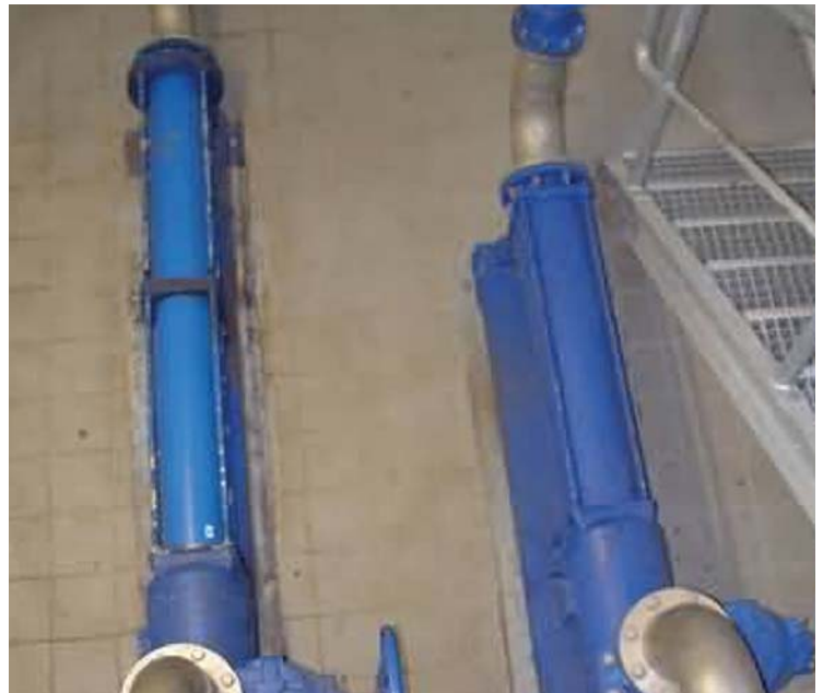
The preliminary filling pump for charging the chamber filter press (right) will be refurbished to make it identical to the existing pump (left).
