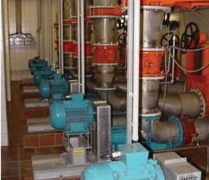
Propeller pumps for recirculation remain unchanged.
