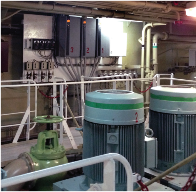
Inside the Maersk Drury engine room, a retro-fit install of the CM-1000 with a 3x50% sea water cooling system.
