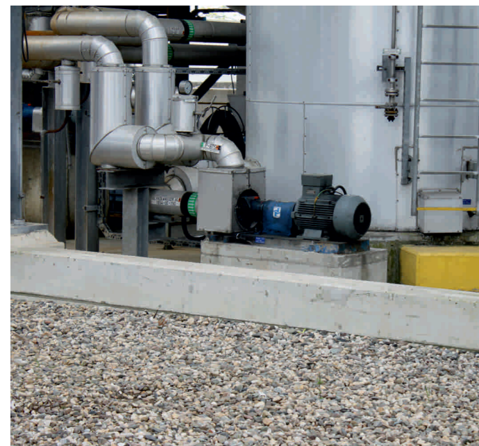
Series CNH-B 50-200G-W20, capacity 60 m 3 /h, liquid glycol/water, process: cooling system.
