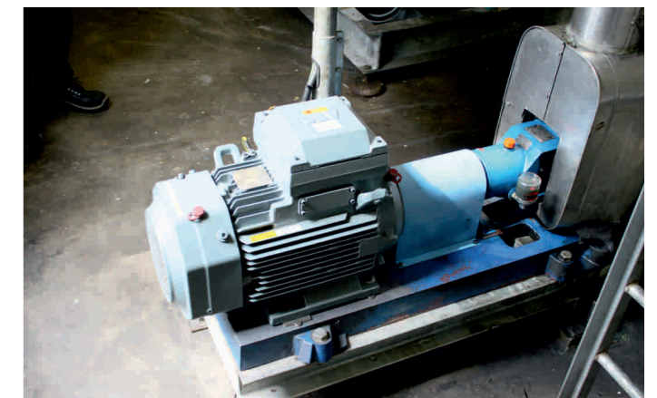
Series CNH-B50-200, capacity 60 m 3 /h, liquid glycol/water, process: cooling system.
